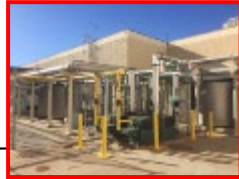
Thermal Energy Storage Plant
